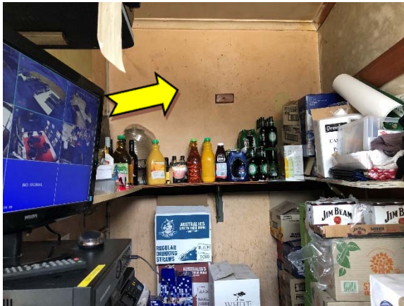
Photo 27. Interior, adjacent bar, storage room, walls – lead-containing cream upper paint systems.
