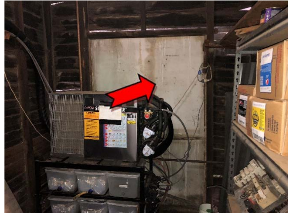
Photo 8. Interior, shed, south-east elevation, infill panels – asbestos-containing fibre cement sheeting.
