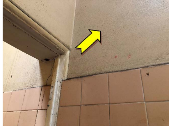
Photo 26. Interior, locker room, toilet and sink area, walls – lead-containing cream upper paint systems.
