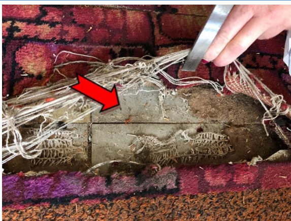
Photo 11. Interior, locker room, under carpet, floor coverings – asbestos-containing vinyl floor tiles.
