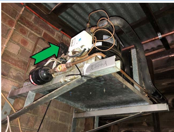
Photo 29. Interior, shed, chiller – Non ODS-containing R410A refrigerant gas.
