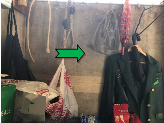
Photo 13. Interior, behind bar, storage area, west elevation, wall – non asbestos-containing fibre cement sheeting.
