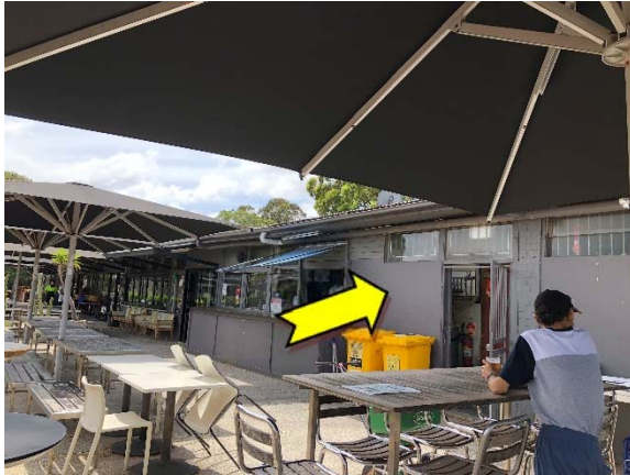
Photo 25. Exterior, throughout, walls – suspected lead-containing grey upper paint systems.
