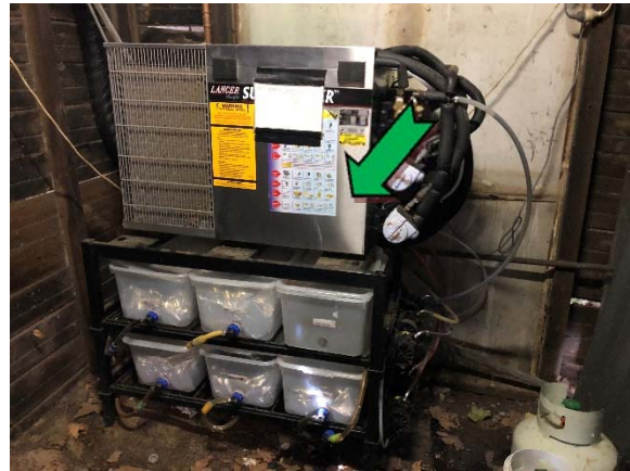
Photo 28. Interior, shed, chiller – Non ODS-containing R134A refrigerant gas.
