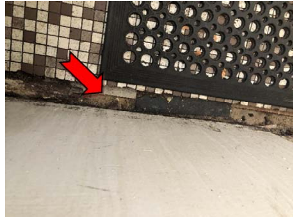
Photo 14. Interior, adjacent bar, on floor, debris – asbestos-containing compressed cement sheeting.
