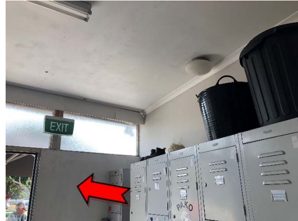
Photo 2. Exterior/interior, locker room, west elevation, walls – asbestos-containing fibre cement sheeting.
