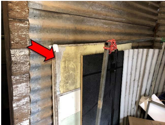
Photo 9. Interior, shed, in front of wall partition, redundant panels – asbestos-containing fibre cement sheeting.
