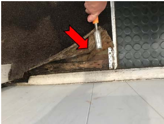
Photo 15. Interior, bar area, beneath carpet, floor coverings (red, blue, yellow, white and black) – assumed asbestos-containing vinyl floor tiles and adhesive.
