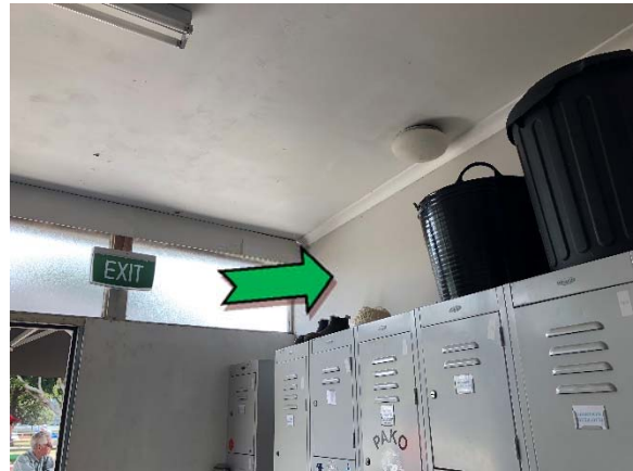
Photo 10. Interior, locker room, north elevation, wall – suspected asbestos-containing fibre cement sheeting.
