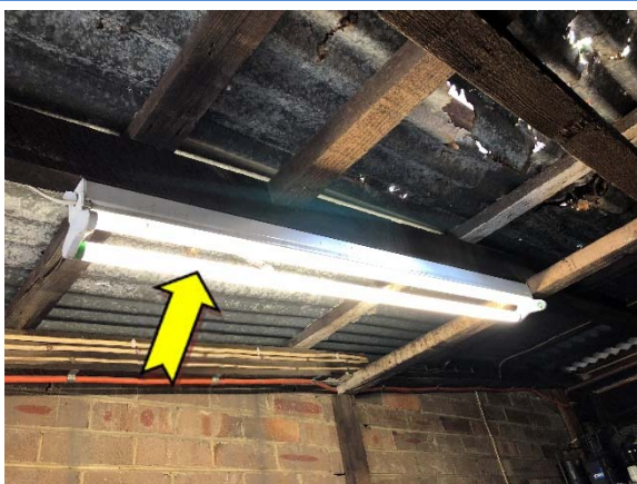
Photo 23. Interior, shed, double tube fluorescent light fitting – suspected PCB-containing capacitors.
