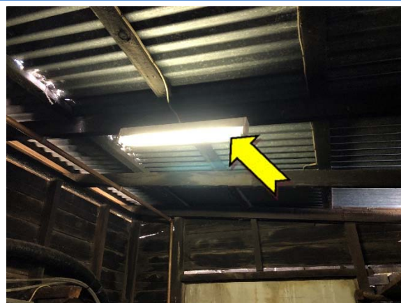
Photo 24. Interior, shed, single tube fluorescent light fitting – suspected PCB-containing capacitors.
